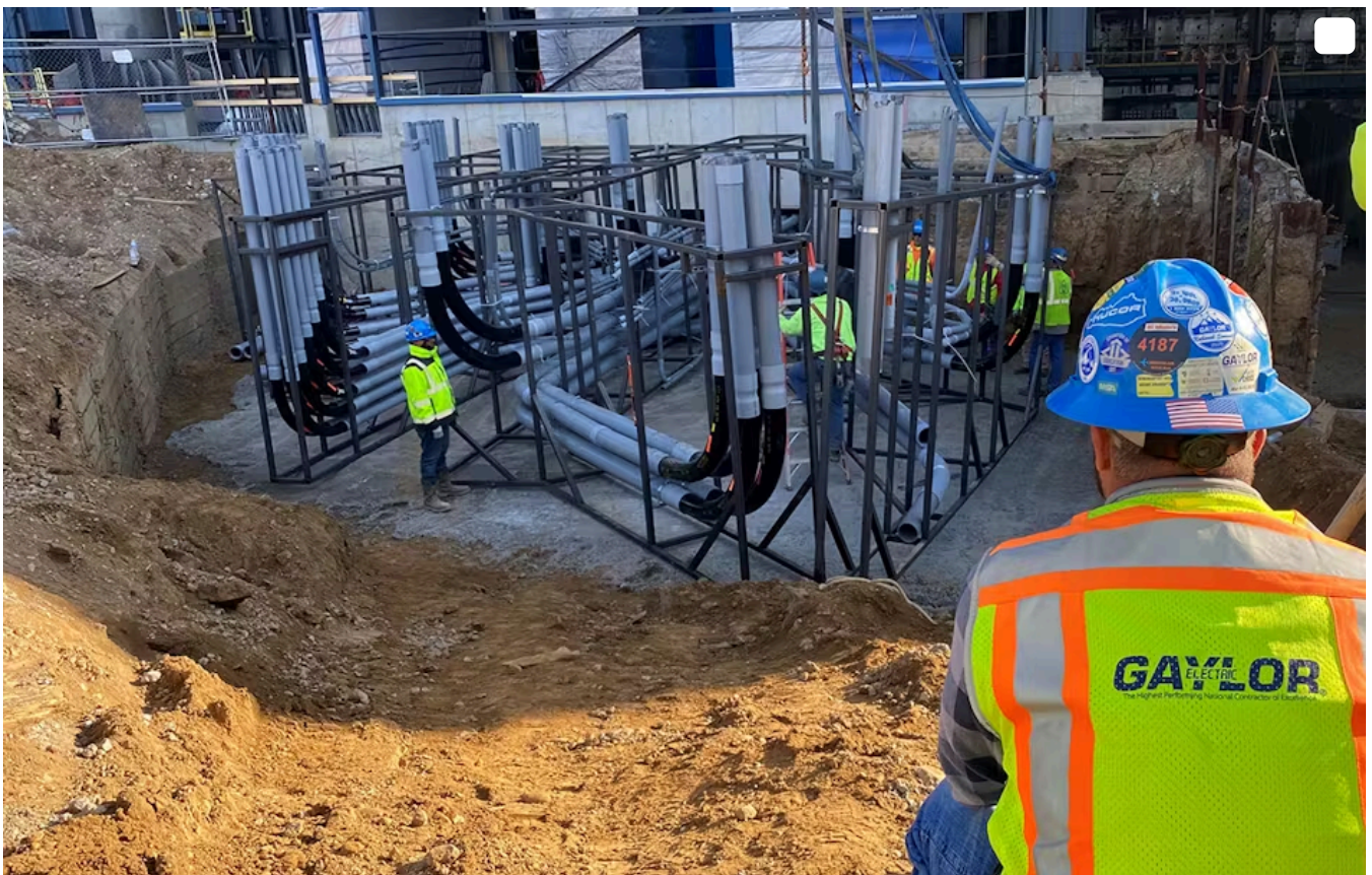
At Nucor Steel, located in Ghent, Ky., the Gaylor Electric team positioned themselves three weeks ahead of schedule by capitalizing on virtual design and manufacturing. The team crane-lifted fully fabricated electrical modules into place.
