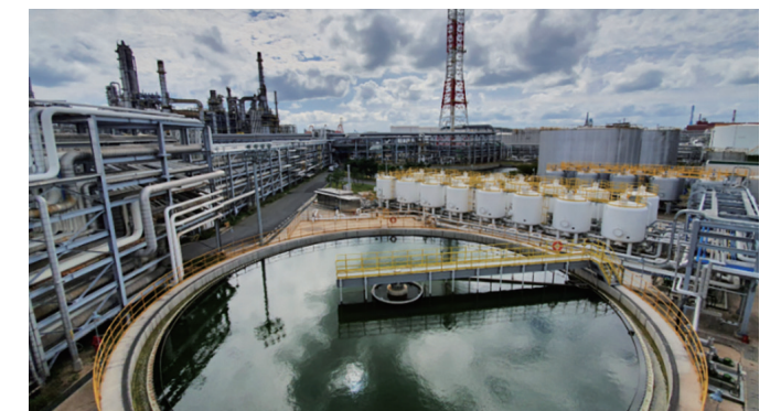
Sedimentation Tank at Wastewater Treatment Plant
