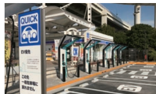
200 kW EV/PHV multi-quick chargers installed in the Daikoku Parking Area
