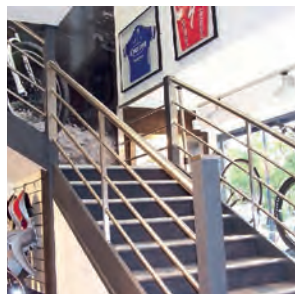
Handrail for retail showroom
