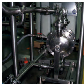
Pump for pharmaceutical process
