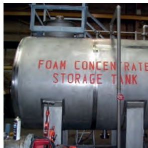
Offshore foam storage tank
