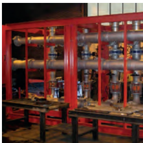
Pipe work skid
